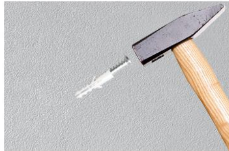
Step 2: Use a hammer to drive the expansion screw into the hole position
